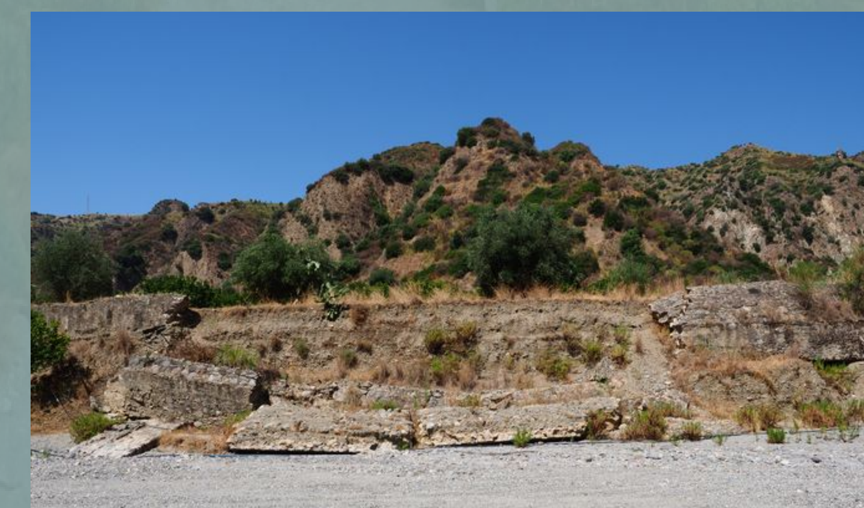
A section of the early 20 th century anti-erosion bulwark at Peristeria, which has been undercut by erosion in recent years.
